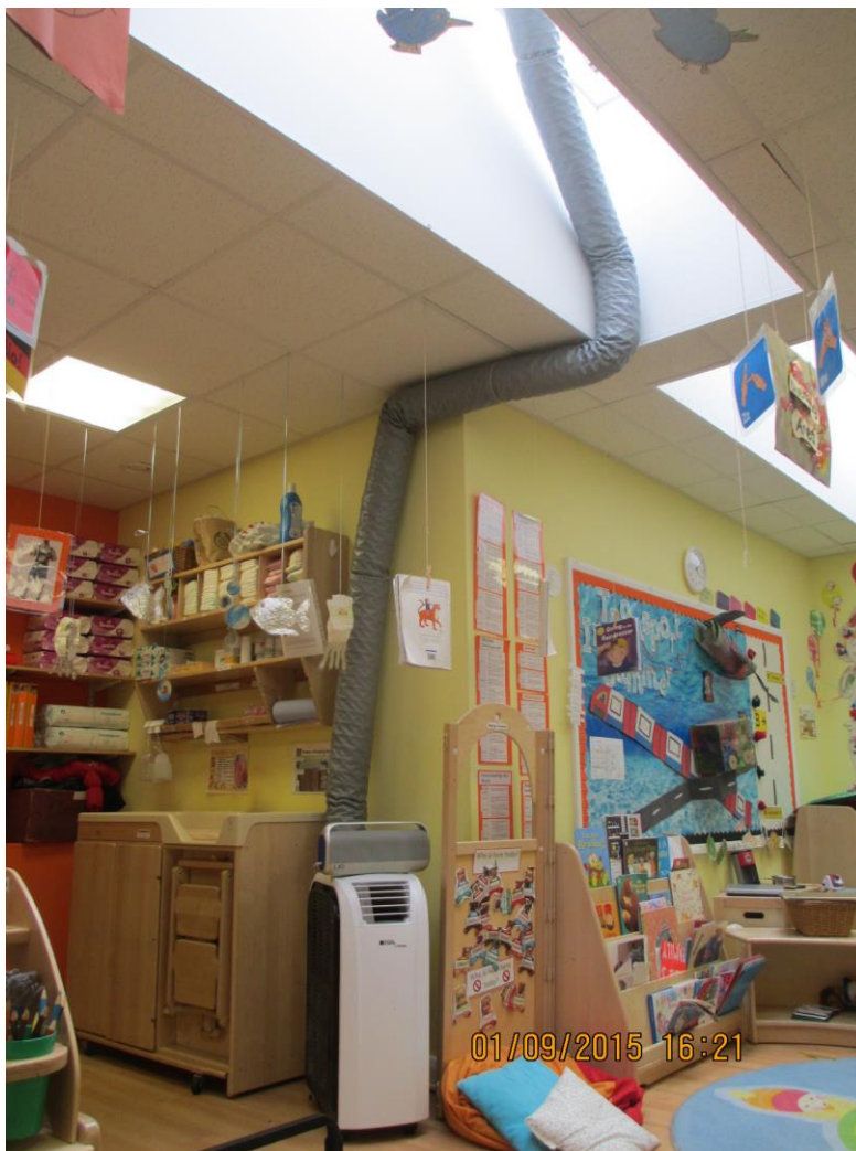
Image 5 – Cooling units currently used inside the nursery.
